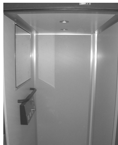
Internal view of the cabin
