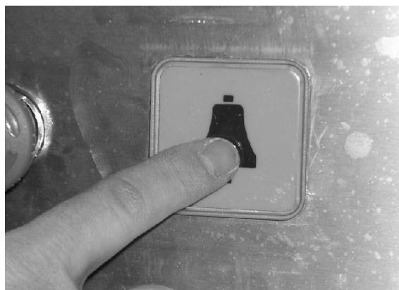
Sonorous alarm activation
