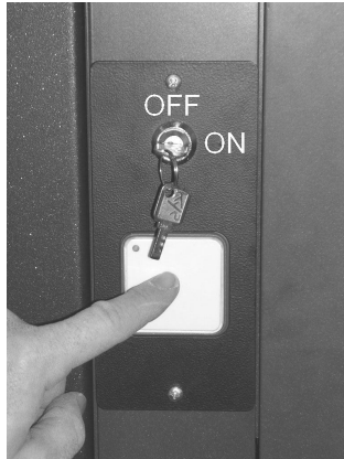
Floor emergency manoeuvre
